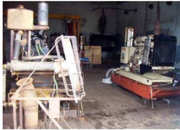
Generators at ELWA
